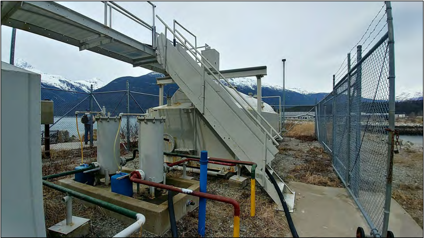
Photograph 3. View of ASTs and piping.
