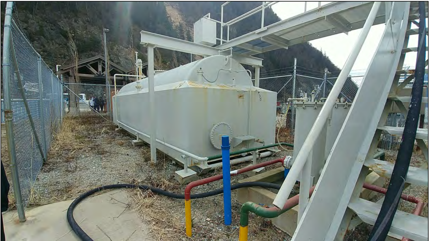
Photograph 4. View of ASTs and piping.
