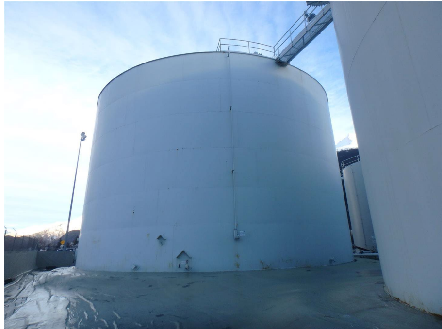
Tank 1 at northwest corner of containment area
