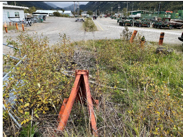
SW end of easement looking NE. This spur line track shows no recent use.
