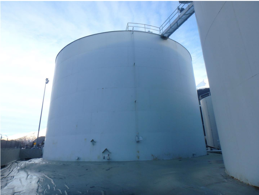
Tank 1 at northwest corner of containment area
