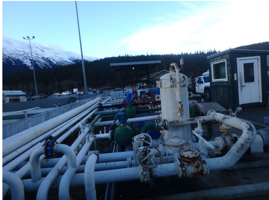
Valves and piping at north end of containment area
