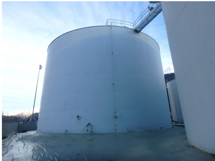
Tank 1 at northwest corner of containment area
