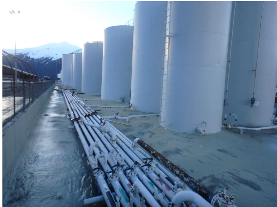
Looking southwest at northeast corner of containment area, tanks 5-11
