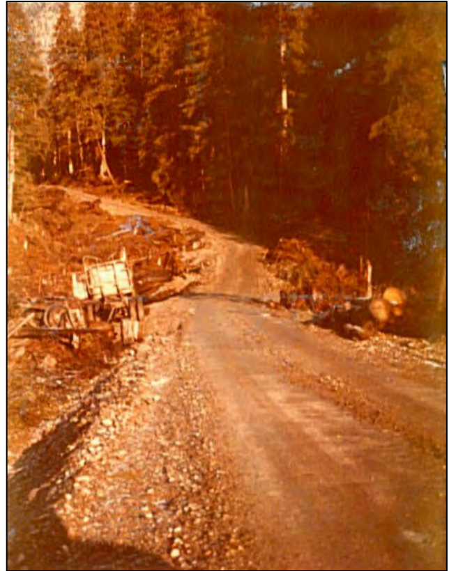
Building West Creek Road and Logging the Area in the 1960's, Photos courtesy of Fred Hosford
