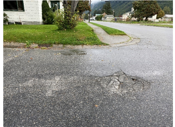
Photo 2 Example of alligator cracking
