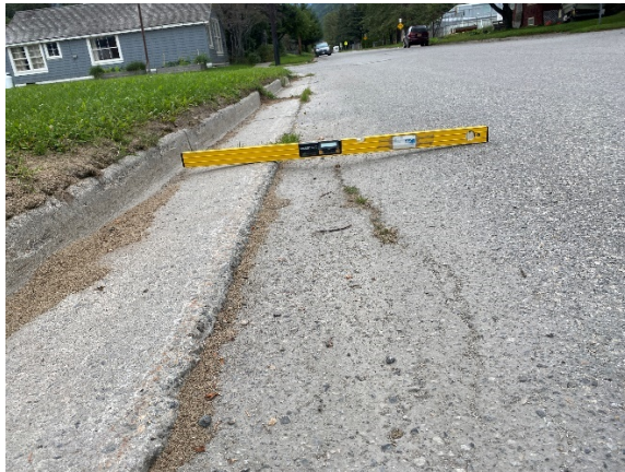
Photo 13 Example of rutting
