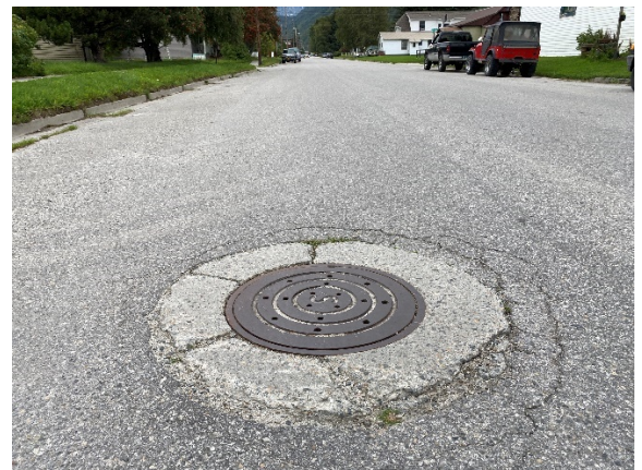
Photo 6 Example of cracked concrete collar around storm drain manhole and surrounding alligator cracking
