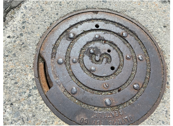
Photo 26 Example of damaged sanitary sewer manhole lid
