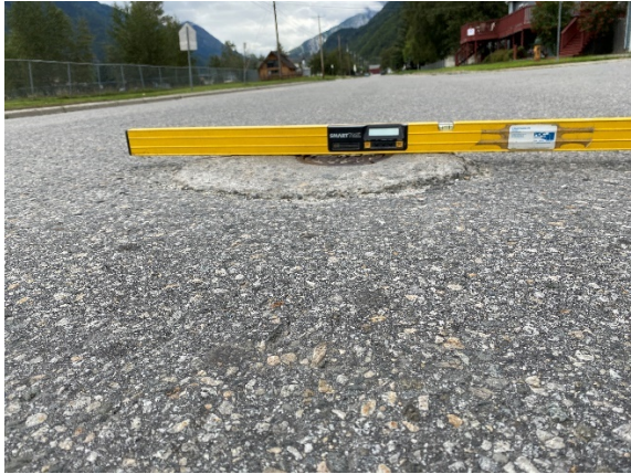
Photo 9 Example of water valve box above grade
