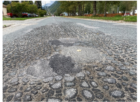
Photo 16 Example of severe alligator cracking and patch work
