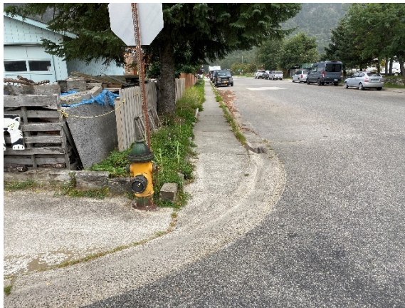
Photo 21 Example of sidewalk curb ramp not meeting ADA standards
