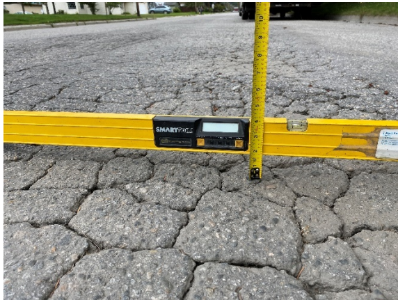
Photo 15 Example of rutting and alligator cracking
