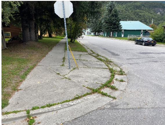
Photo 19 Example of concrete sidewalk cracking
