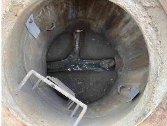
Photo 25 Example of sanitary sewer manhole with infiltration
