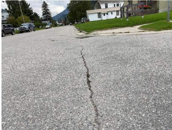
Photo 1 Example of a pavement joint failure
