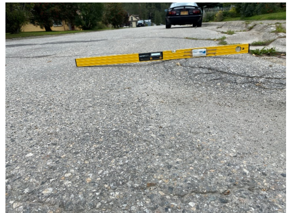
Photo 12 Example of heaving.
