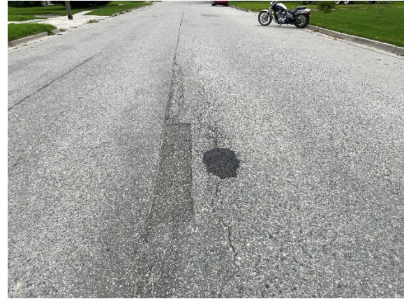
Photo 10 Example of longitudinal cracking and patch work
