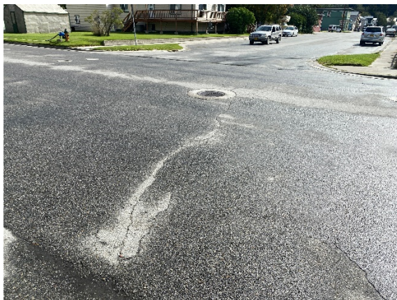
Photo 5 Example of transverse cracking
