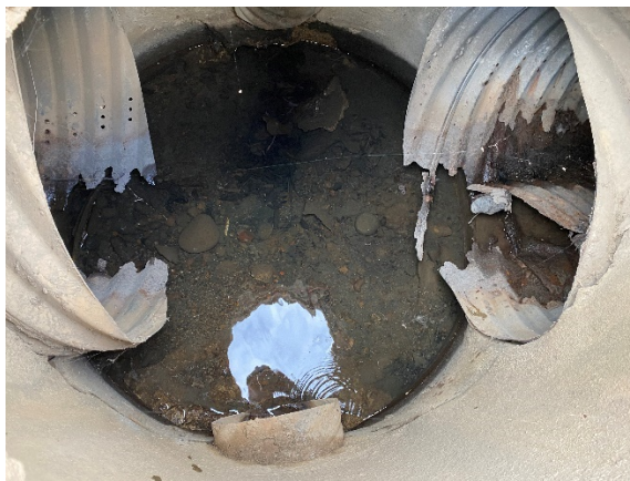
Photo 23 Example of corroding storm drain pipes
