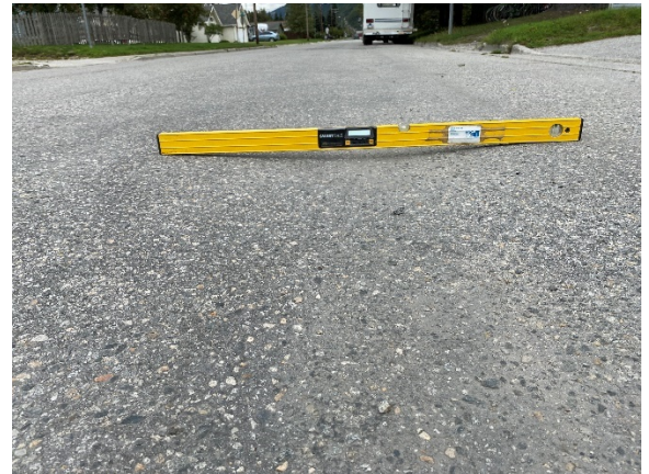
Photo 14 Example of rutting
