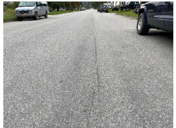
Photo 4 Example of longitudinal cracking
