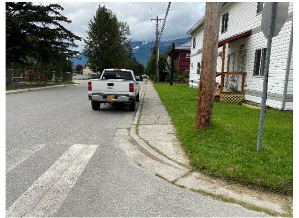
Photo 22 Example of concrete sidewalk not meeting ADA standards
