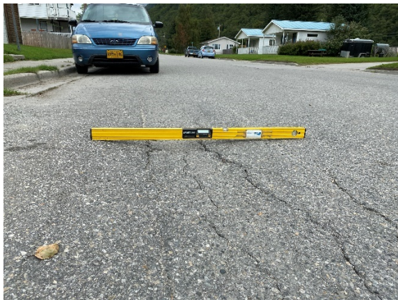
Photo 17 Example of rutting and longitudinal cracking
