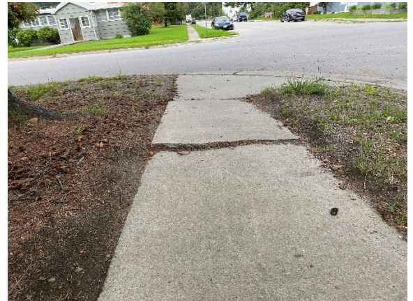
Photo 20 Example of concrete sidewalk cracking and heaving
