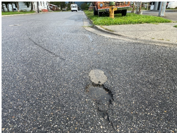
Photo 3 Example of a pothole
