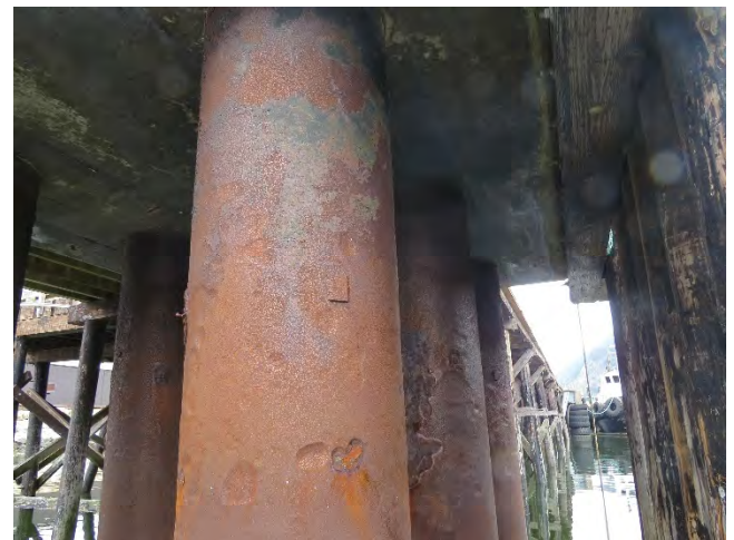
Photo 87- Large pitting at ore dolphin piles (2 of 2)
