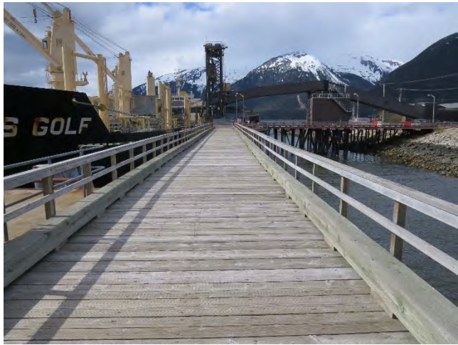
Photo 88- Decking surface condition
