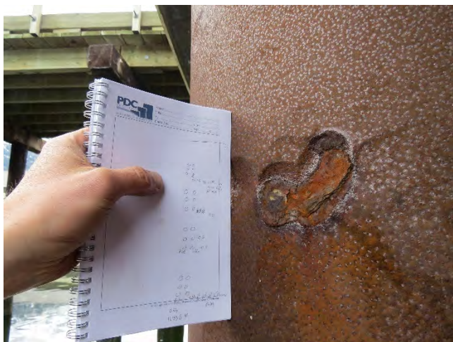
Photo 86- Large pitting at ore dolphin piles (1 of 2)
