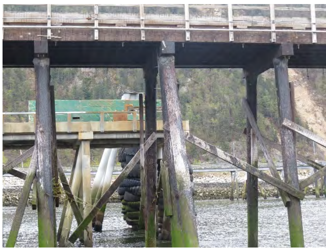
Photo 82- Broken cross-bracing (1 of 2)
