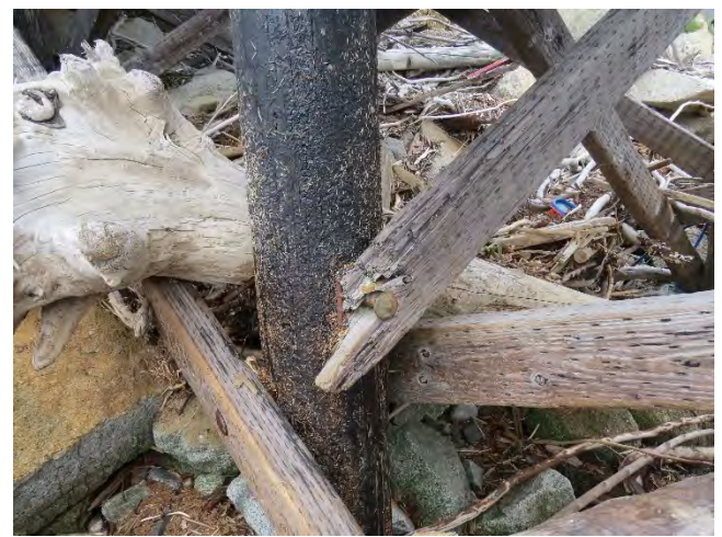
Photo 83- Broken cross-bracing (2 of 2)
