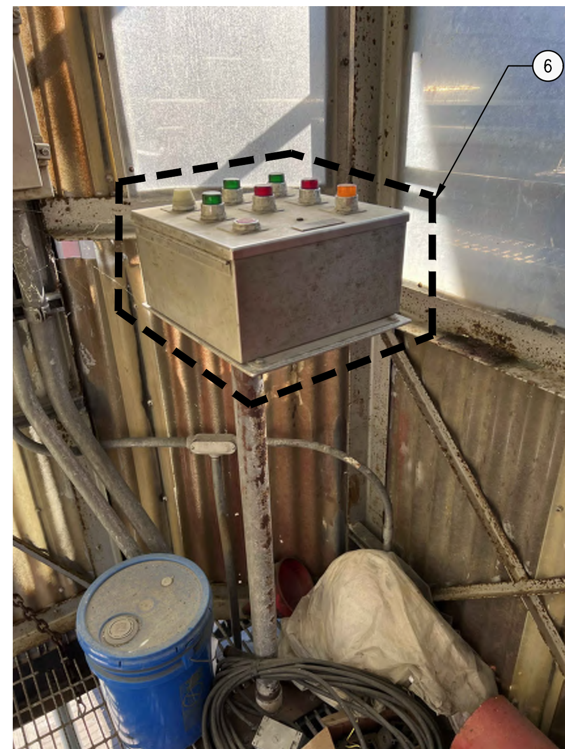
7 D2.20 DEMO SHIP LOADER BOOM CONTROL PANEL
