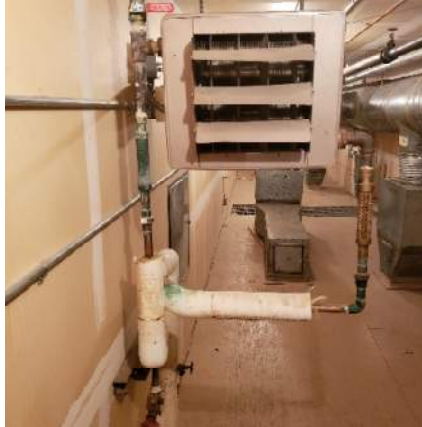
Dissimilar Metal Corrosion
