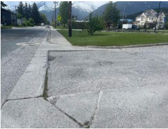
Photo 1 – Worn asphalt pavement at entrance
