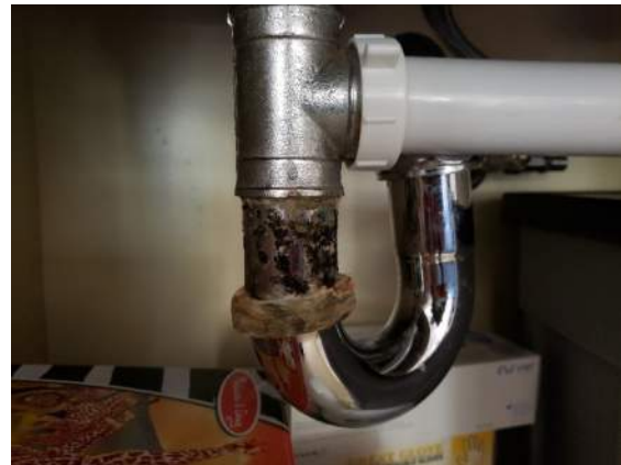
Classroom 315 Sink P-Trap
