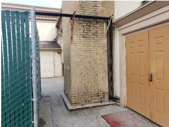
Exterior Fuel Oil Piping
