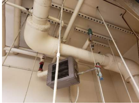
Boiler Room Unit Heater
