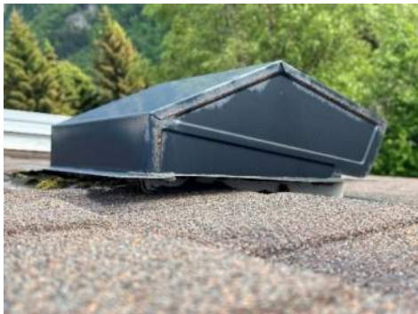
Photo A32 - Reroof 3:12 slope, improper penetration
