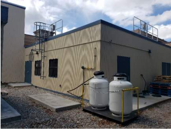
Kitchen Propane System
