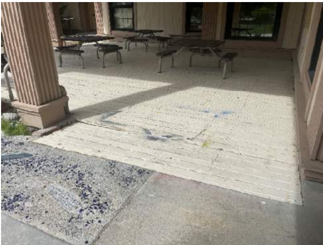
Photo AE25a - Deck to be replaced.
