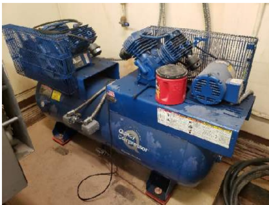
Pneumatic Control Air Compressor
