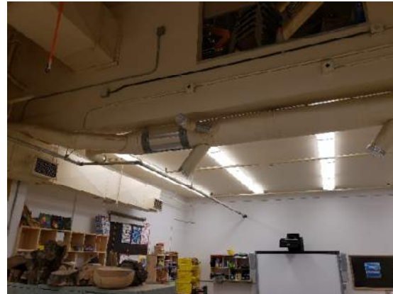
Dust Collection System
