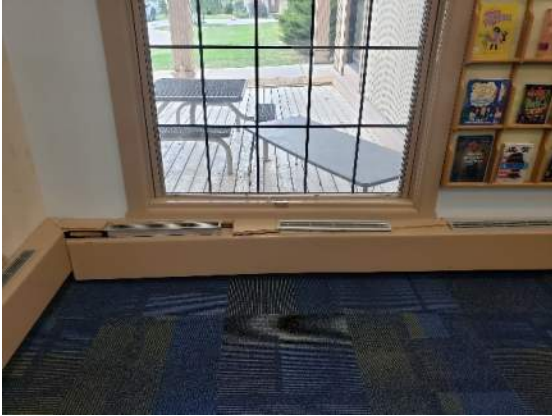
Damaged Fintube Enclosure (Library)
