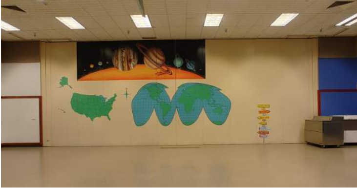
AI03 – Operable partition in Multi-Purpose Room
