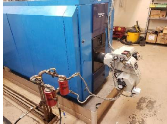
Water Heater Fuel Oil Piping
