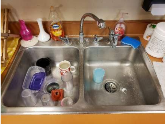
Typical Classroom Sink
