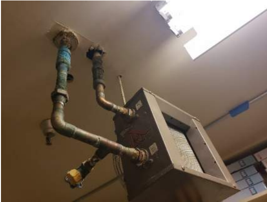
Unit Heater Flex Oxidation
