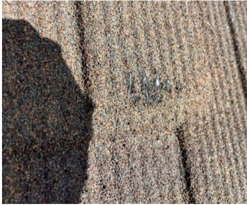
Photo AE28 - Reroof 3:12 slope, surface wear
