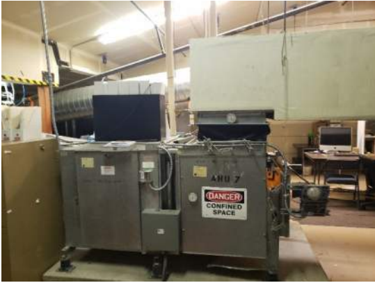
AHU-7 Return Air Smoke Detector
