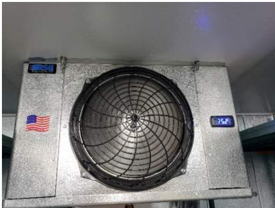
Kitchen Refrigerator Evaporator
