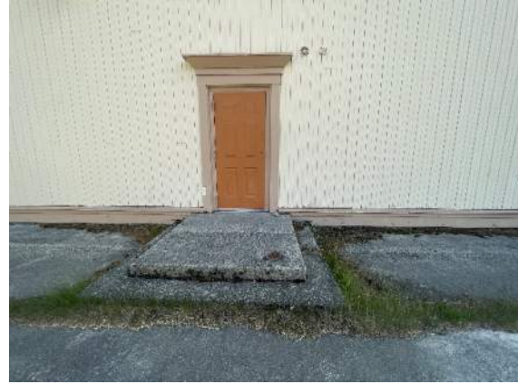
Photo 33 – Mainline valve/ valve box in concrete step
