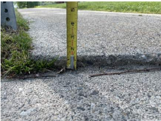
Photo 8 – Raised sidewalk panel
