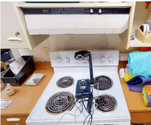
Kitchen 10B Range Hood
