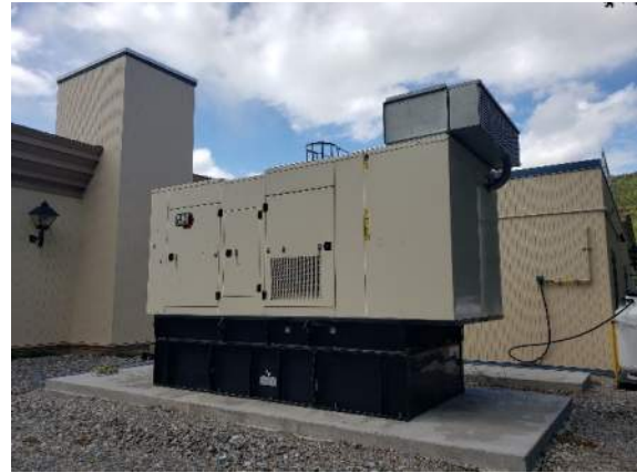
Generator Subbase Fuel Tank
