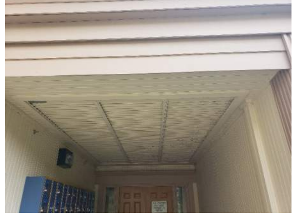
Exterior Louver in Entry
