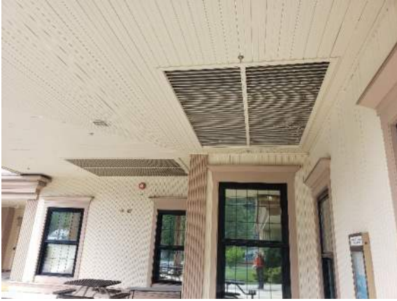
Exterior Louvers in Canopy
