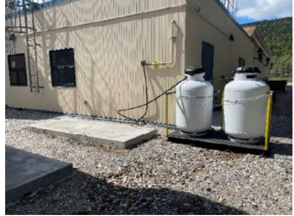
Photo 22 – Propane tank storage
