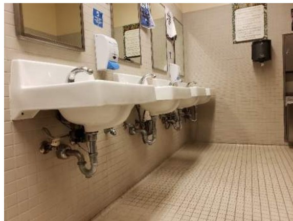
Typical Restroom Lavatory
