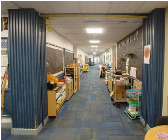
A116 – Pneumatic Gate at Hallway 100B
