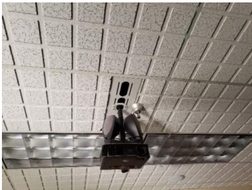
Sprinkler Head Above Projector
