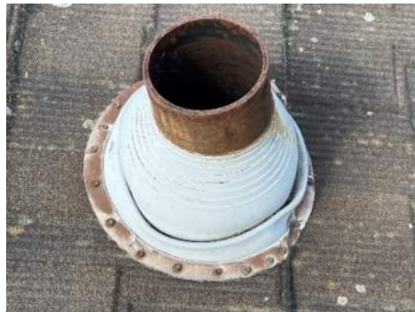
Photo A33 - Reroof 3:12 slope, improper penetration
