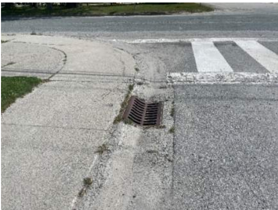
Photo 25 – Worn crosswalk striping
