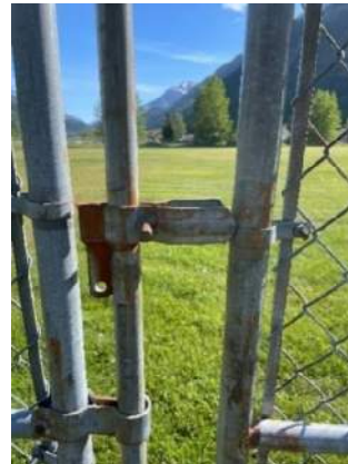
Photo 18 – Typical gate latch gap
