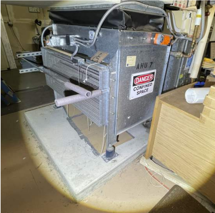
Photo 44 — Typical mezzanine level housekeeping pad and mechanical equipment.
