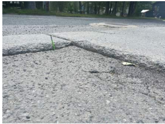
Photo 2 – Close up of worn asphalt surface
