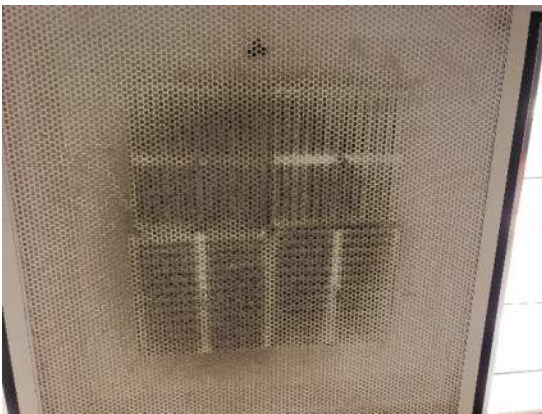
Classroom 9B Return Air Grille
