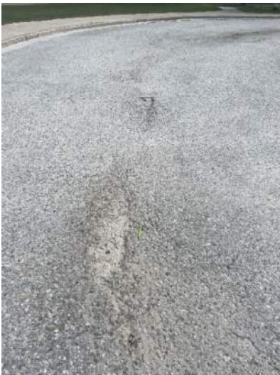
Photo 3 – Asphalt deterioration on driveway
