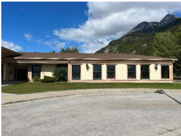
Photo AE01– East wing south wall – greatest exposure
