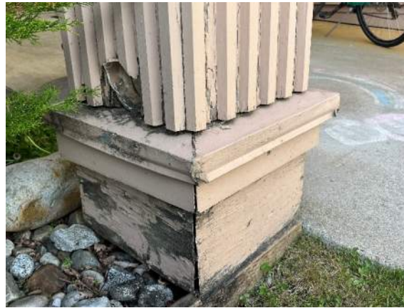
Photo AE09– Orig ext fin cap at canopy – column enc water
