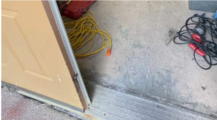
Photo 41 — Spalling at interior slab-on-grade (Boiler Room).
