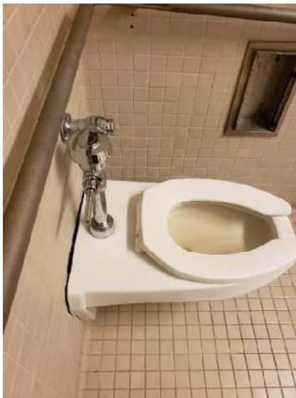
Boy’s Restroom Toilet Wall Separation
