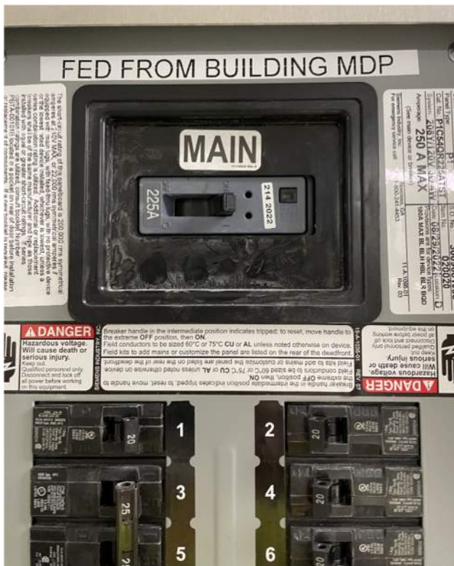
Note from Drawings (above), Kitchen electrical panel
