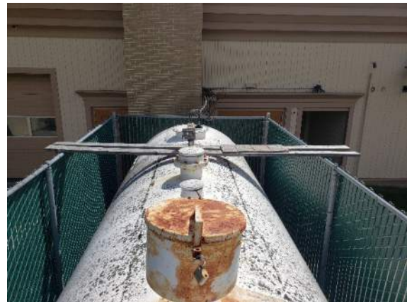
Fuel Storage Tank
