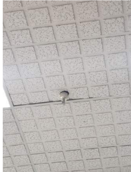
Sprinkler Head Missing Escutcheon
