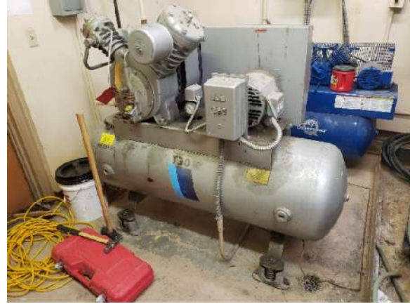
Fire Sprinkler & Shop Compressor
