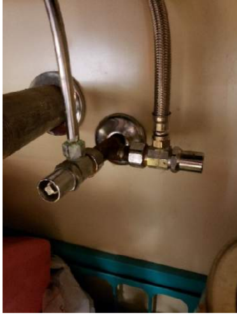
Angle Stop Valve Corrosion
