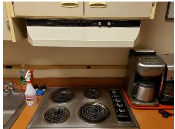
Break Room 22 Range Hood
