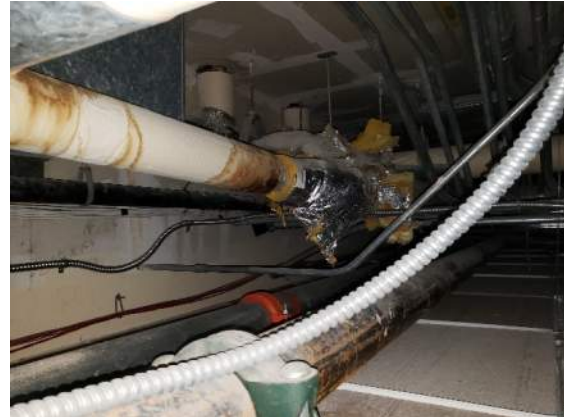
Hydronic Mains Old Leak
