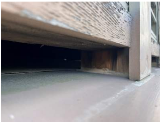
Photo AE36 - Cupola, open flashing joint and vert penetration w/ sealant
