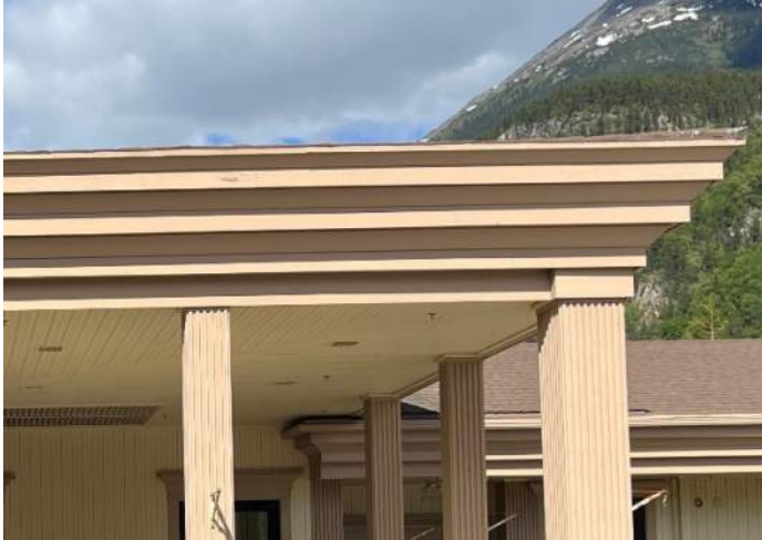
Photo AE10– Orig wood soffit/fascia, typ
