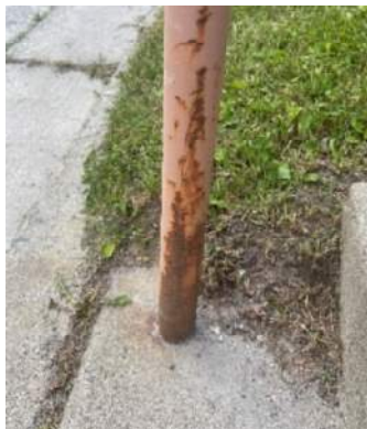
Photo 12 – Close up of handrail corrosion
