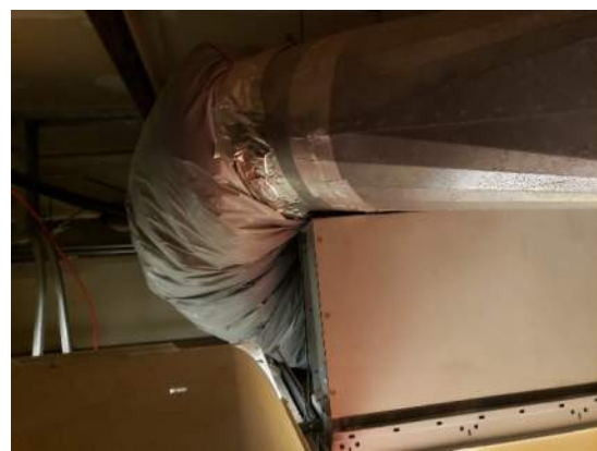
Storage 10B Flex Duct Connection
