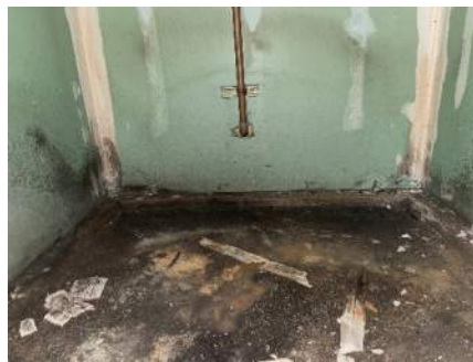
Photo AE05a – Moldy interior of chase
