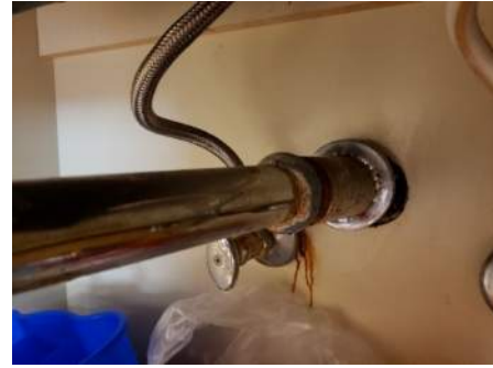
Previous Leak at Wall Penetration
