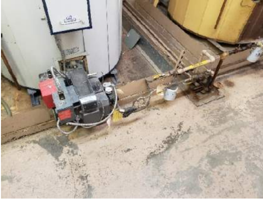
Boiler Fuel Oil Piping
