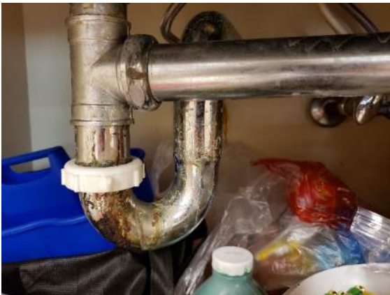
Classroom 301 Sink P-Trap
