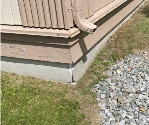
Photo 39 — Damaged foundation insulation and flashing.
