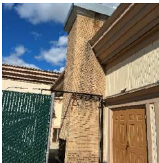
Photo AE05 – Orig brick veneer at south chase
