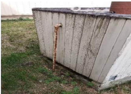
Science Lab Propane Piping
