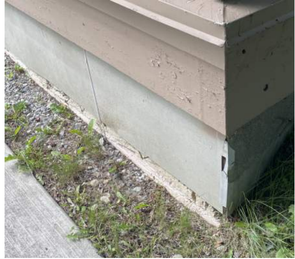
Photo 40 — Damaged foundation insulation and flashing.
