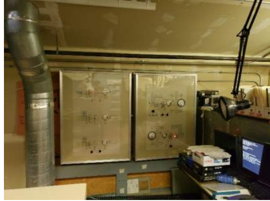
AHU Pneumatic Control Panels
