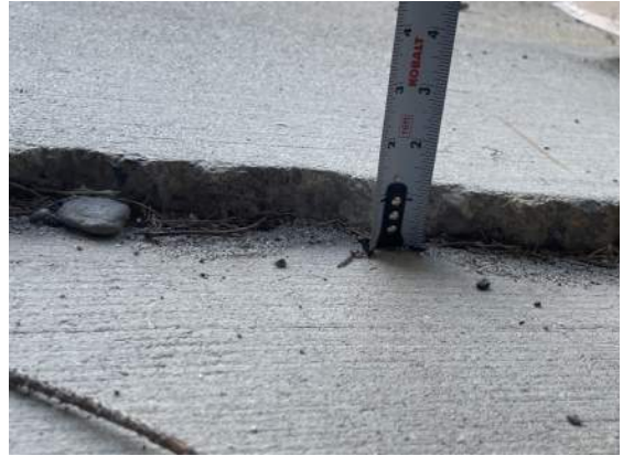
Photo 42 — Significant cracking at exterior slab near door 125.
