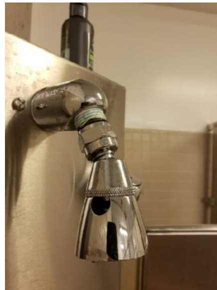
Showerhead Missing Valve Handle
