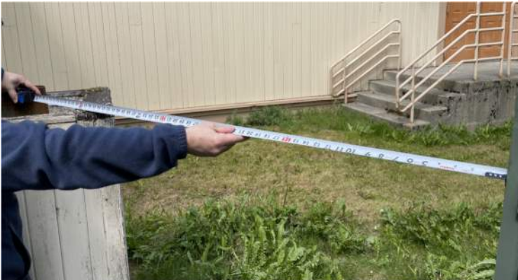
Distance between the Transformer Propane Tank
