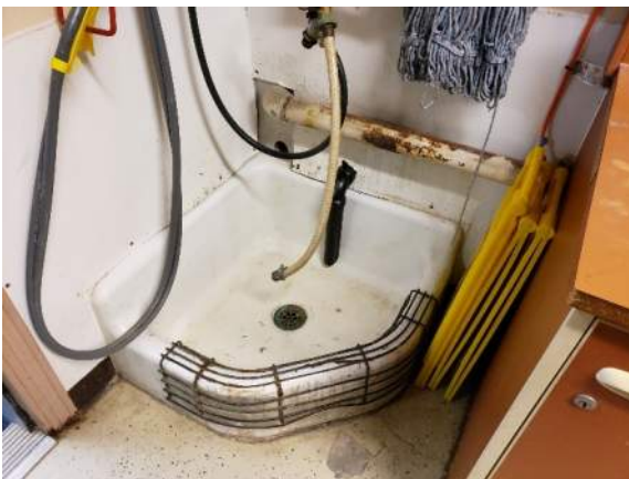
Janitor Mop Sink Drain Line w/o Air Gap
