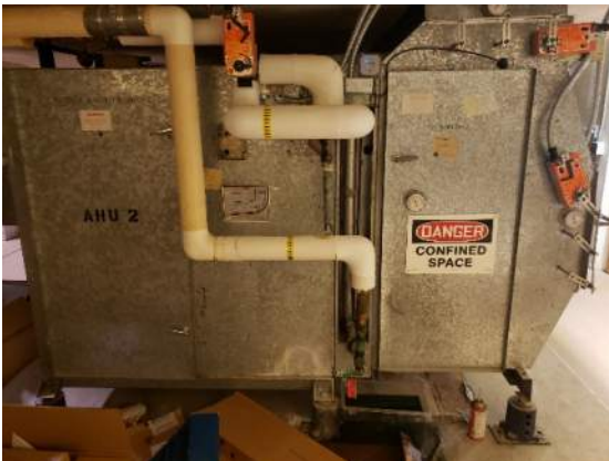
AHU-2 Heating Coil Leak
