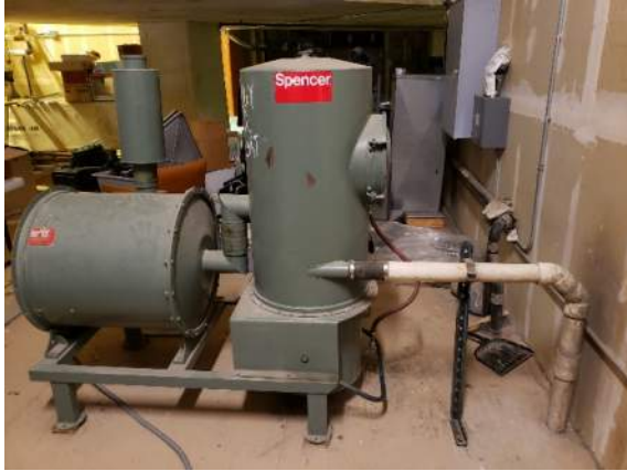
Central Vacuum System
