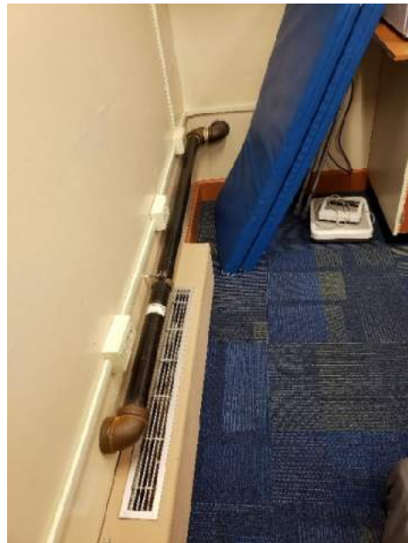
Exposed Sprinkler Drain Line
