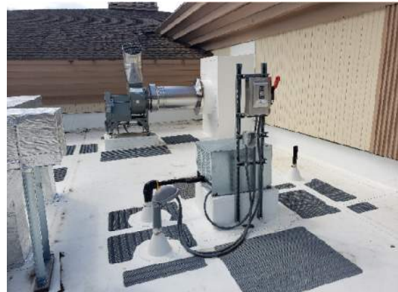
Kitchen Refrigerator Condenser
