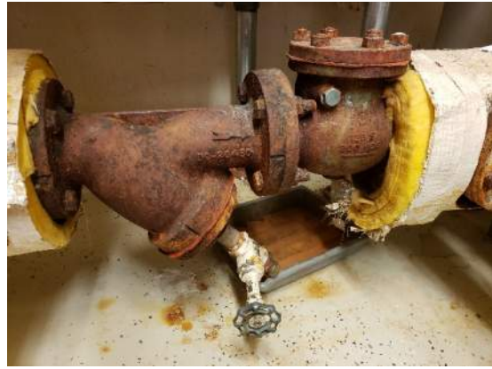
Rusting Strainer & Check Valve
