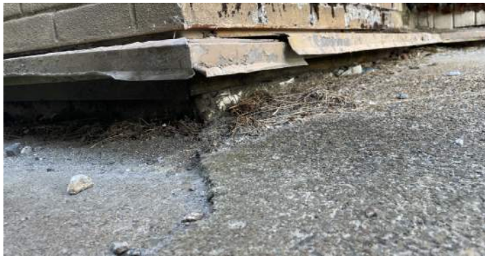
Photo 43 — Typical settlement and spalling of exterior slabs.
