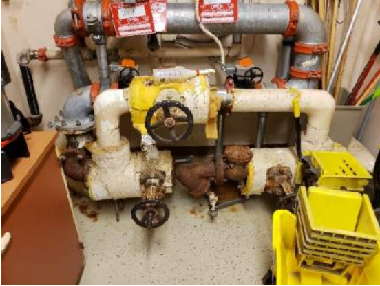
Water Service Entrance
