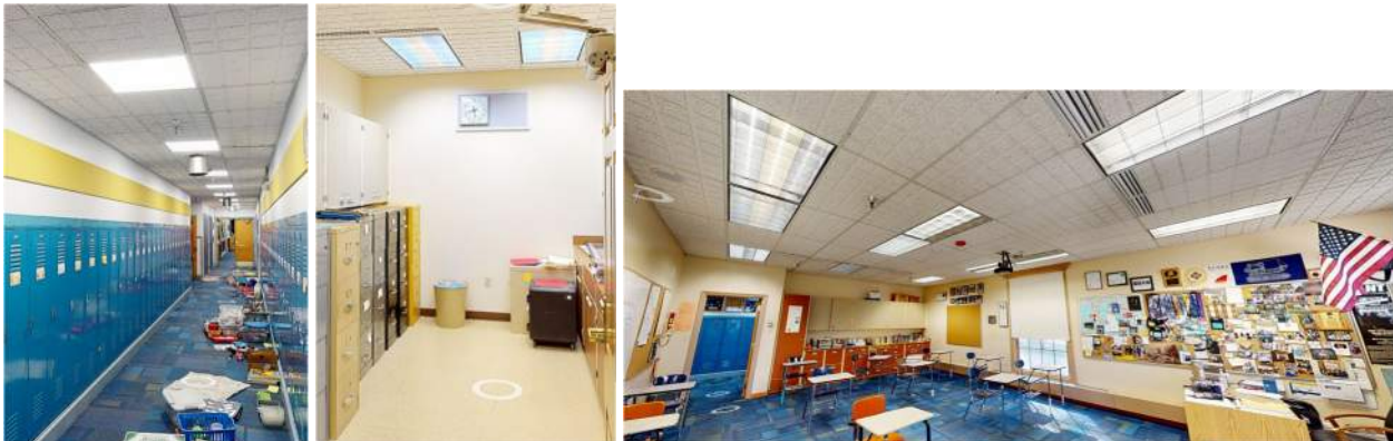
Left to Right: Hallway with new LED lighting, Storage Room with Ex. 2'x4' fluorescent lights, Classroom with Ex. 2'x4' fluorescent lights
