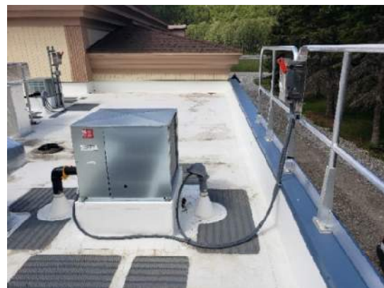
Kitchen Freezer Condenser
