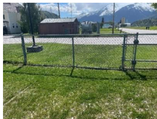
Photo 20 – Inoperable playground rolling gate
