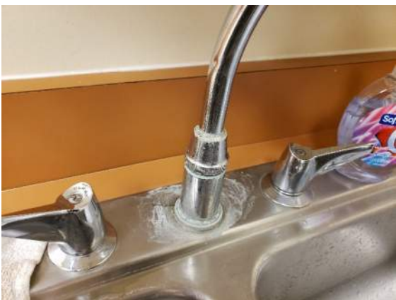
Storage 10A Sink Corrosion
