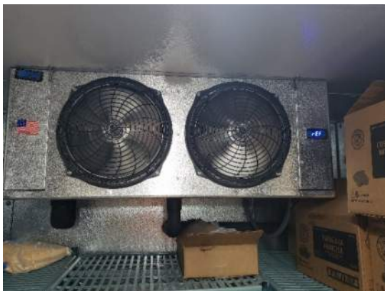
Kitchen Freezer Evaporator
