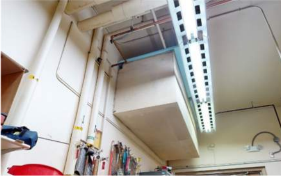
Boiler Room Relief Air Opening
