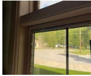
Photo AE13– Orig window, failed IGU seals, typ
