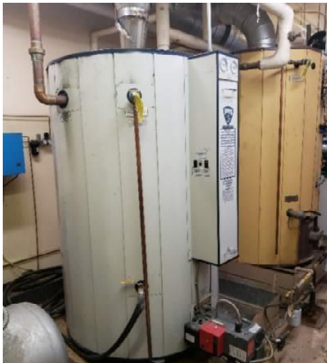
Water Heater & PRV
