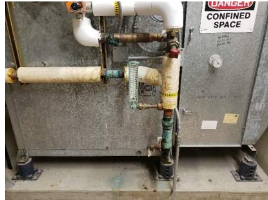
AHU-5 Heating Coil Oxidation
