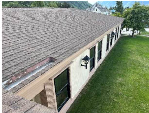
Photo AE38 – Built in gutter, otherwise no gutters except in limited applications
